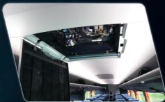
Standardized power stations making component identification easier.
